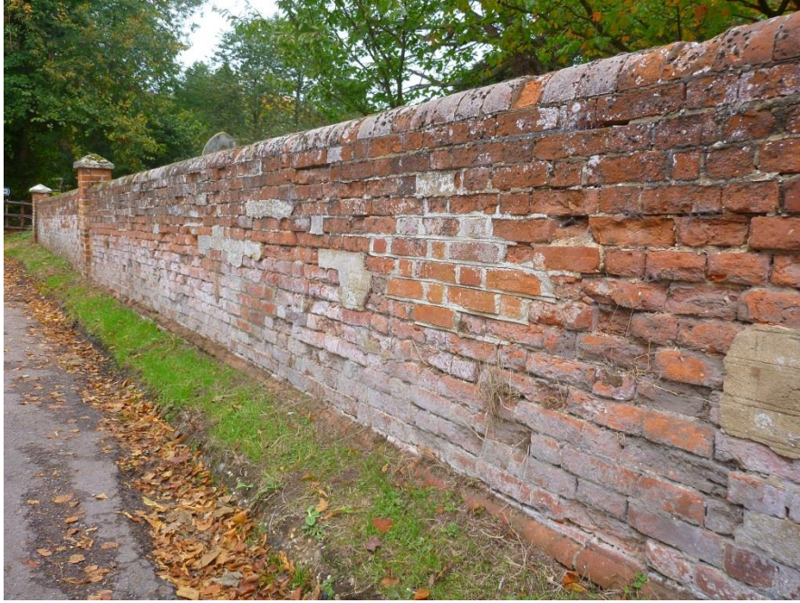
Fig. 51: Brick wall outside the Church of Saint Mary the Virgin. It is in need of repairs.
