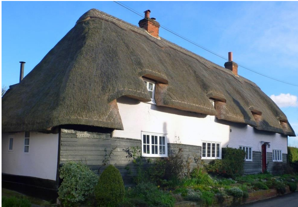
Fig. 18: Thatch End C18th timber-framed cottage, formerly four cottages. Plastered with low level weatherboarding. Half-hipped thatched roof. Ground floor and attics, with a single-storey outshut to northern end. Two brick chimney stacks and small brick outbuildings to rear.
