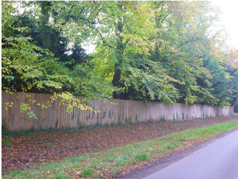
Fig. 74: The fence along The Street to the North of Furneaux Pelham Hall does not form a positive welcome to the Conservation Area boundary from the West. The owner should be encouraged to plant a mixed native hedge in front of the fence to hide it or reduce its impact in views along The Street.
