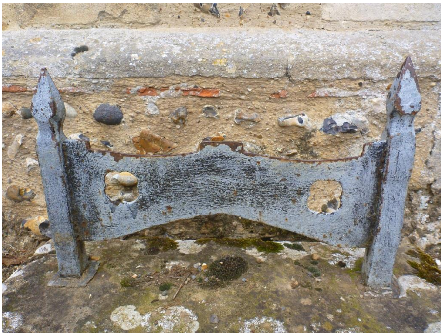
Fig. 61: Decorative cast iron foot-scraper outside the Church of Saint Mary the Virgin. It and other foot-scrappers are in need of painting.
